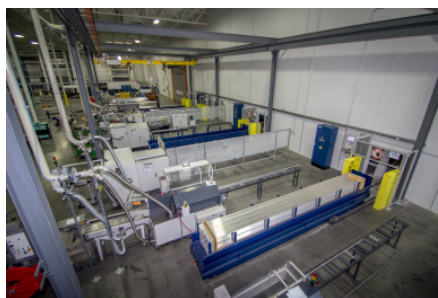
The longspan shelving store uses four retrieval stations to supply the linked-up saws over short distances.
