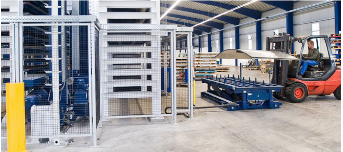
The scissor lift table at the input/output station is equipped with loading pins and insertable stops for setting up a corner coordinate system, allowing precise alignment of the sheets.
